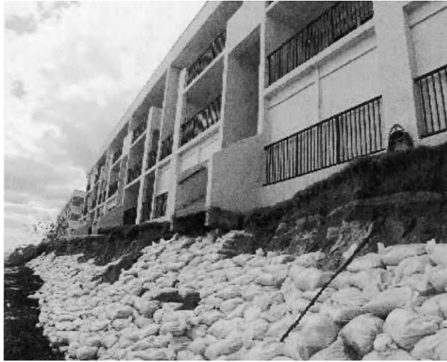
FIGURE 12-1 Florida hotel faces risk of beach erosion from Hurricane Irene. Courtesy: Ty Harrington/FEMA.
