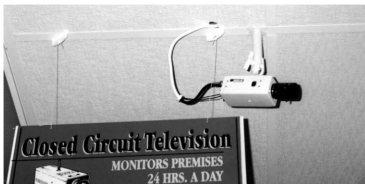
FIGURE 7-18 Closed-circuit television (CCTV) sign. Camera at top.
