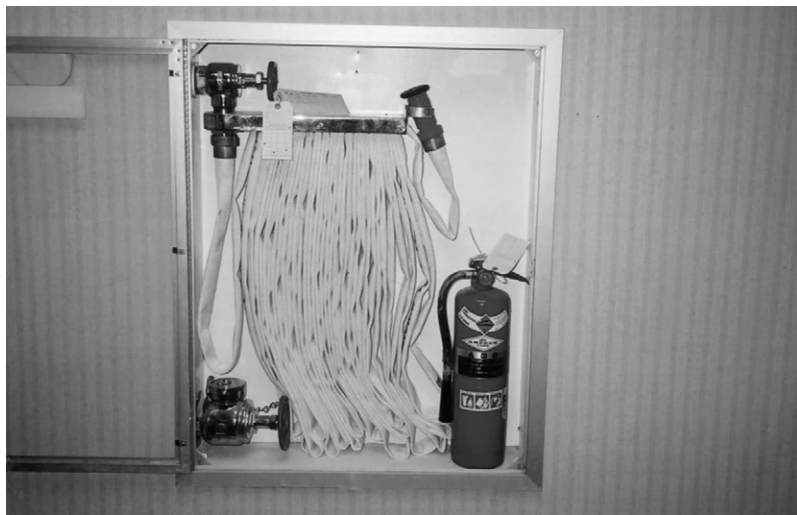
FIGURE 13-5 Standpipe system including wall cabinet, hose with nozzle, and valves. A portable fire extinguisher is also contained in the cabinet.
